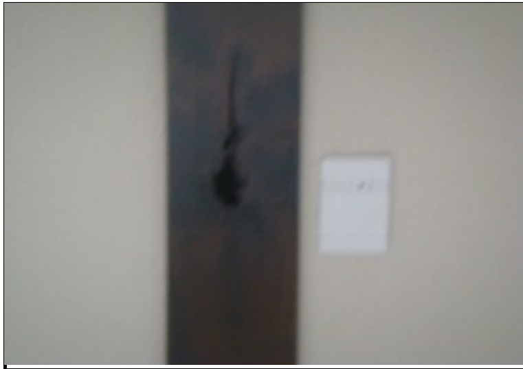
Large size knot at ceiling wood trim (off the kitchen area).
