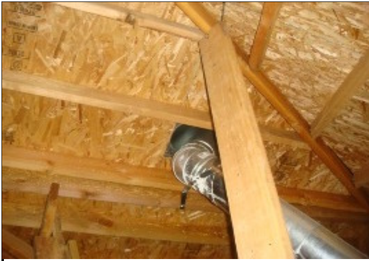
Attic -- Recommend to seal areas where the furnace flues are venting across the roof (found evidence of prior water penetration).
