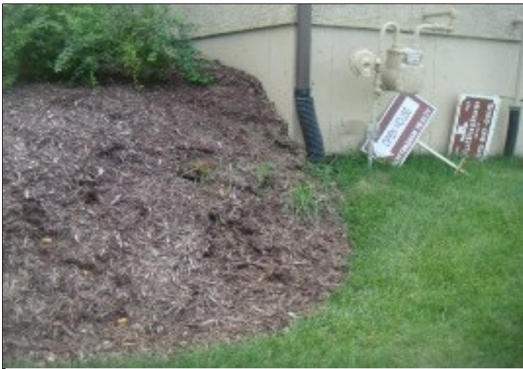
Retaining Walls -- Recommend to build a retaining wall at the front-right corner of the building (lots of soil erosion, surface right now is covered with mulch).
